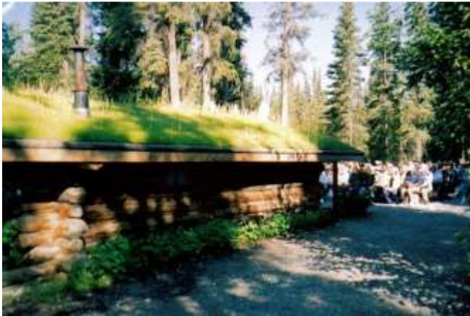
Sod roof... needs cutting!!
